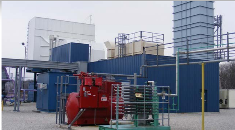
Peaking Power Plant owned and operated by Wolverine Power Co-op, MI
